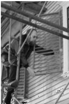
Project manager Charlie Allen (at left); John Mazzeo (below left) pulls paper from a roll of ice and water shield. The new rear chimney is visible above him.
